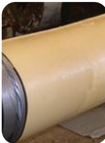
Field Joint Coating System Comprised of Raychem Heat Shring Sleeves, Cuming Half Shells, and Floatec 6000 Materials
